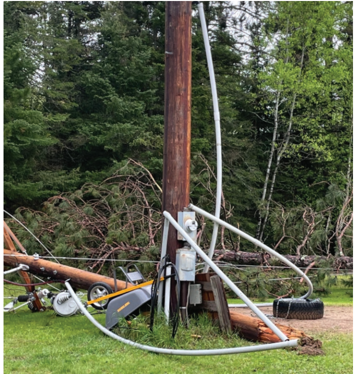
FD&L enables LCP to quickly react to poles downed by storms, like the one pictured above.
