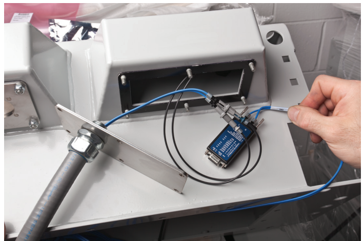
Fig. 2 - Zero-voltage close waveforms being downloaded from the SmartClose capacitor switch with fiber-optic cable.
