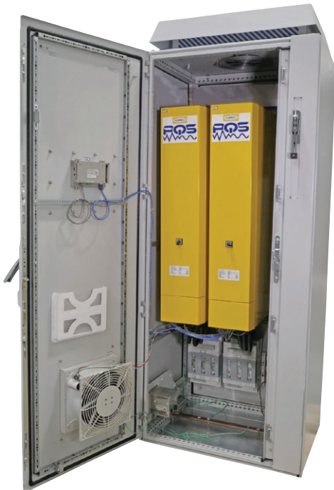
Figure 6: AHF 380V 60Hz 100A located at 2AHF-2A panel
