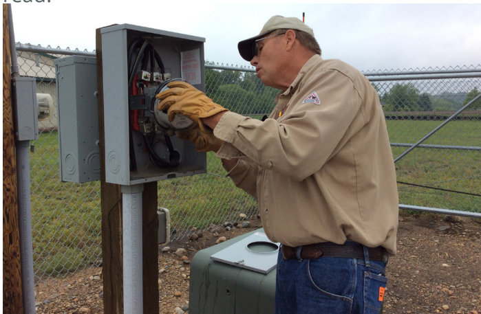
Fig. 2- Runestone Electric Association managed the changeover from its previous AMI system to TWACS with internal resources.
