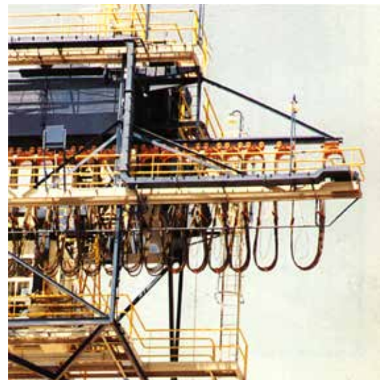
ON THE COVER: Typical Gleason I-beam festoon system providing power and control to a crane.
