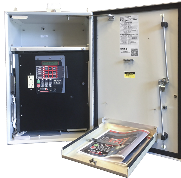
Figure 3 M-2979 Recloser Control Cabinet
