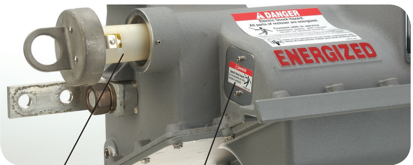
Battery bayonet partially removed from recloser
