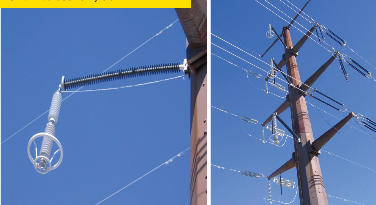
345kV - Wisconsin, USA
