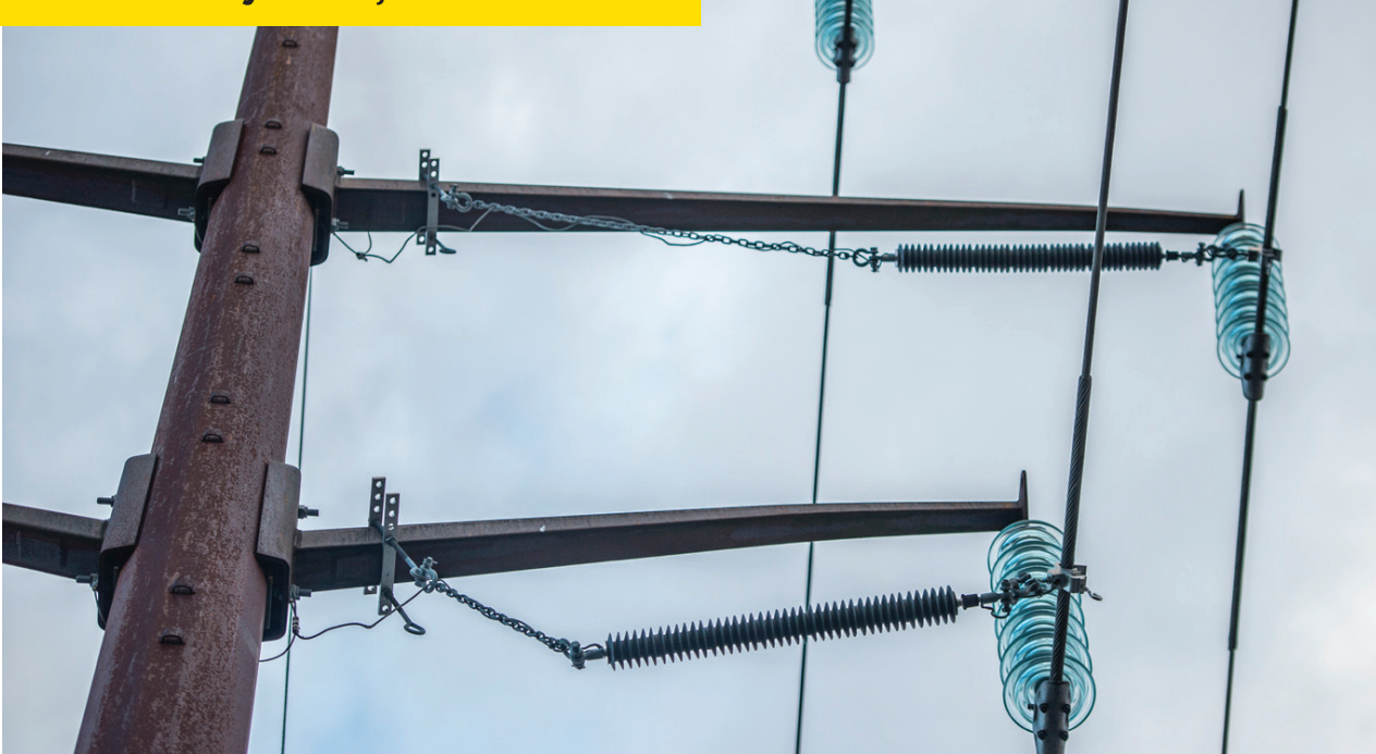
69kV - Pennsylvania, USA
