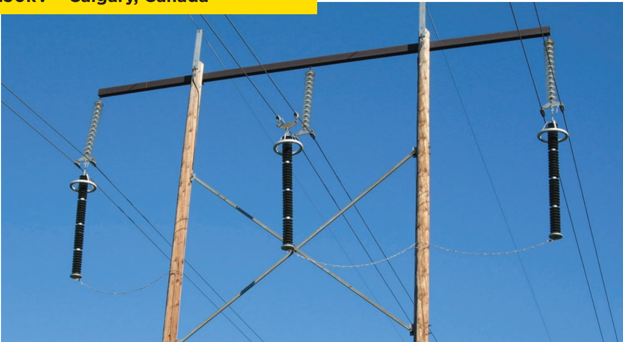
230kV - Calgary, Canada
