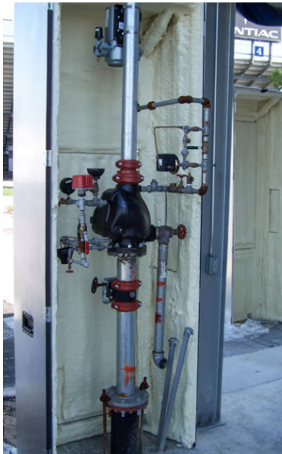
Custom Enclosure - Gainesville Speedway
