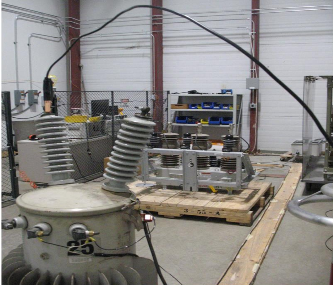
SSAO transformer setup
