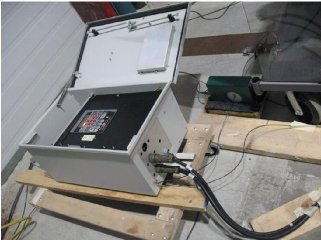
Beckwith control connection in SSAO test
