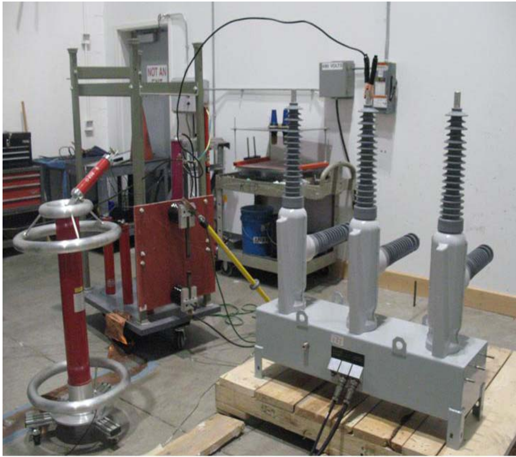
SSAO Recloser Setup
