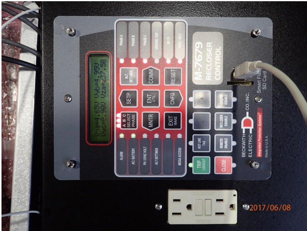
Figure 17: Overall view of the tested recloser controller.
