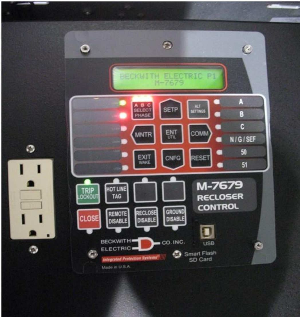
Beckwith control screen display
