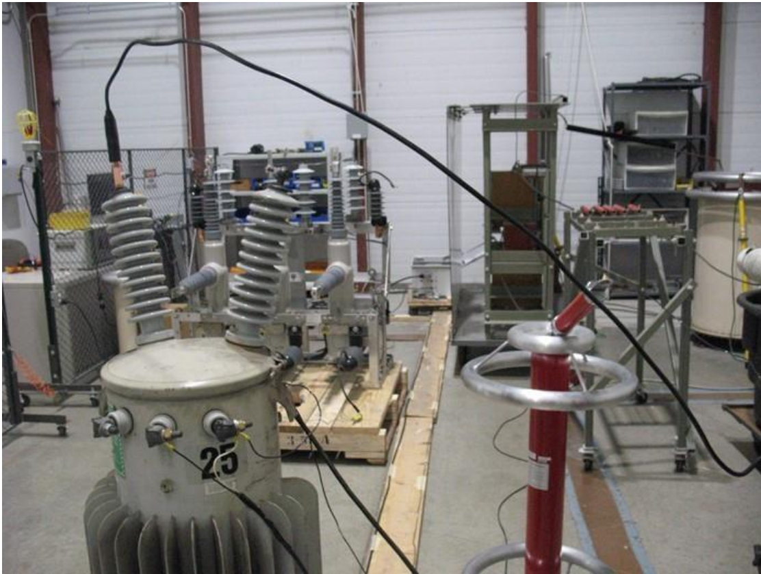
SSAO Transformer test setup
