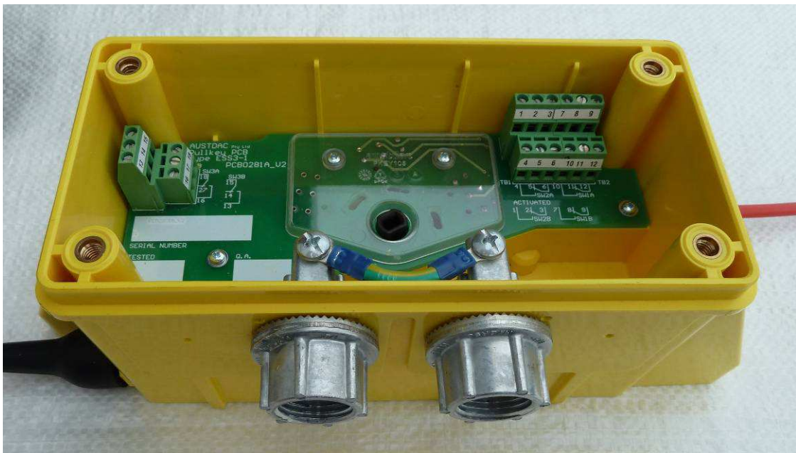
Photograph 10 Earth continuity of conduit hubs
