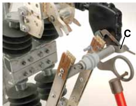
C. Load disconnect blade opens through interrupter.
