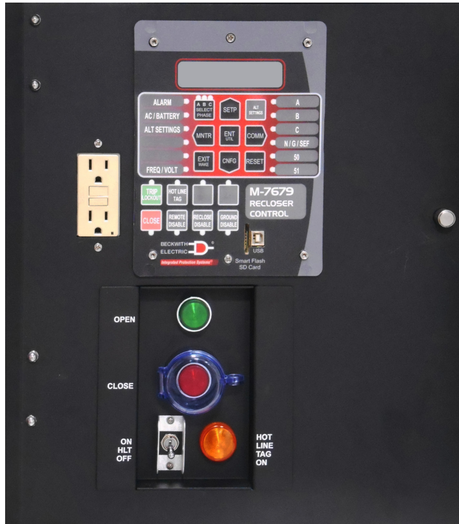
Figure 2 External Trip/Close with Hot Line Tag Assembly in M-2979 Custom Swing Panel
