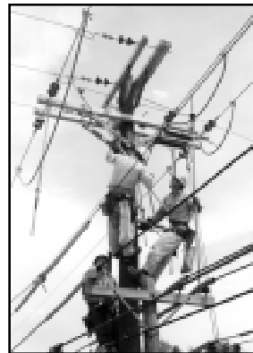
Right, phasing test to determine B to B phase.
