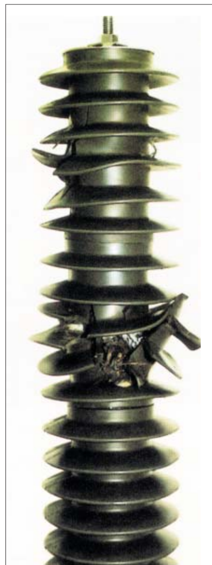
A three-unit Protecta*Lite surge arrester with its polymer-housed epoxy/fiberglass wrapped metal-oxide disc modules ruptured to relieve internal pressure generated by a fault current arc of 10,000 amps for 10 cycles. Note the polymer housing has been split open, but the housing remains attached.
