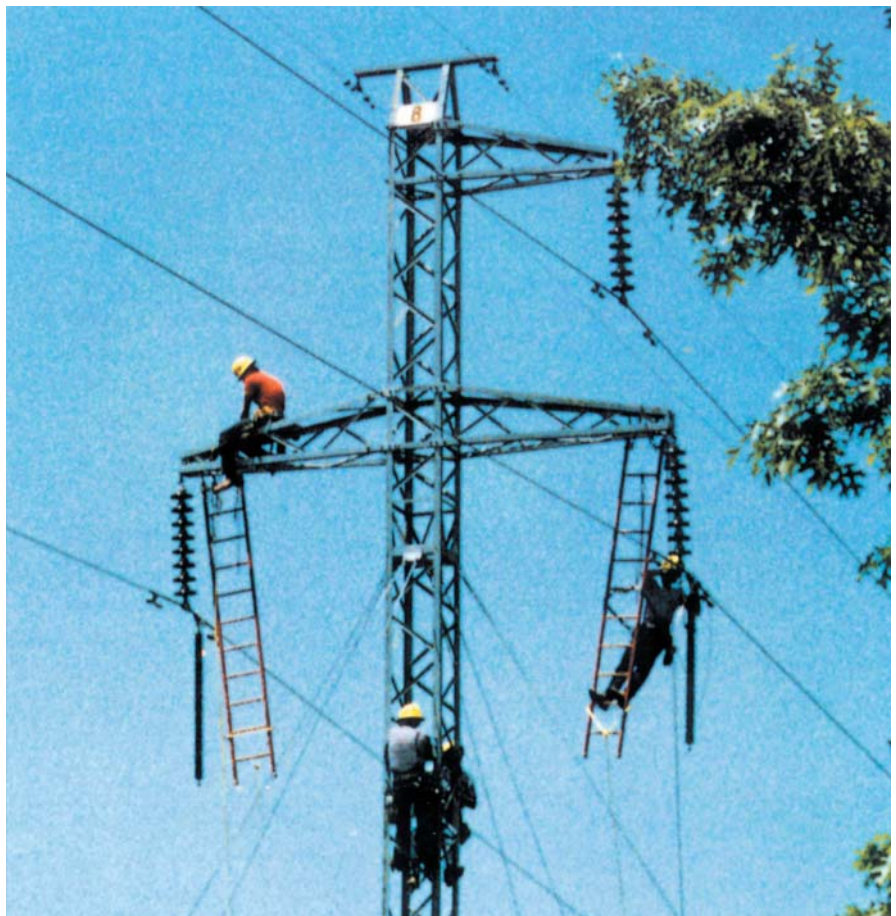
Protecta*Lite arresters, which weigh only 35 lbs., are installed below line insulators.
