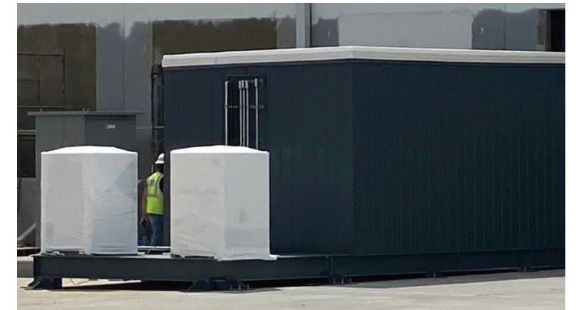
Modular Data Center
