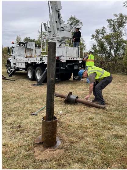
Photo 1: Installation at Centralia, MO Site
