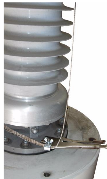
Figure 7 : Ground fixing on bushing bottom with the grip wrench and the Ground Tape.
