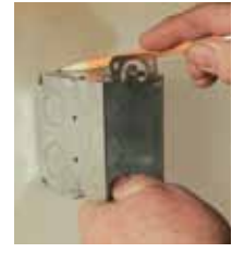
Trace outline of the box on the wall in an area with no obstructions (framing, wiring, pipes, etc.)
