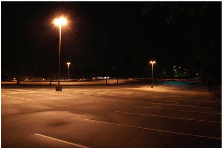
400w HPS units, double configuration, mounted at 28 ft.
