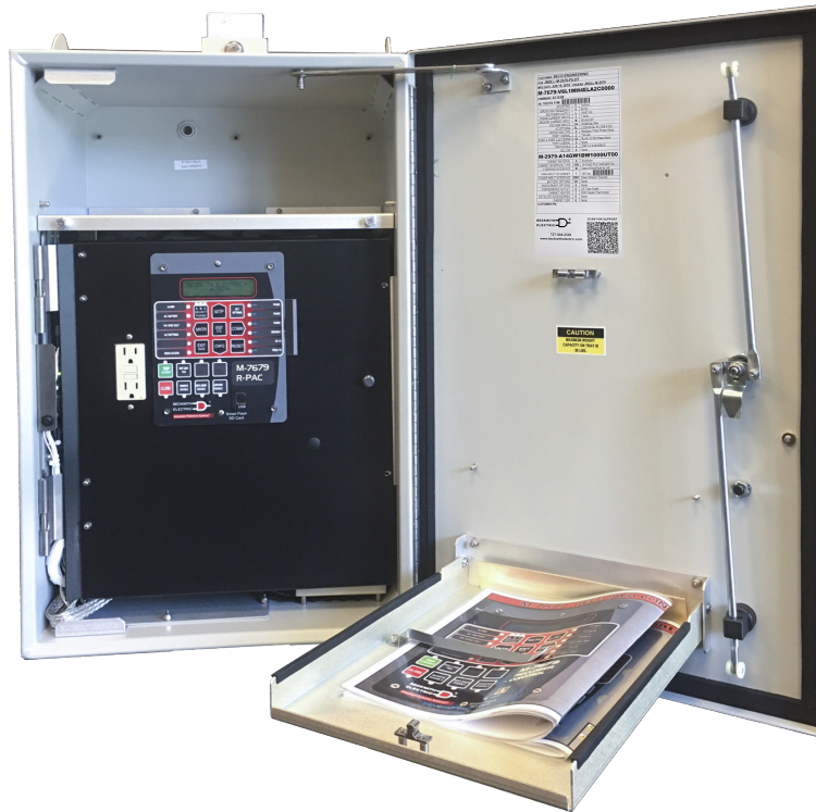
Figure 3 M-2979 Recloser Control Cabinet
