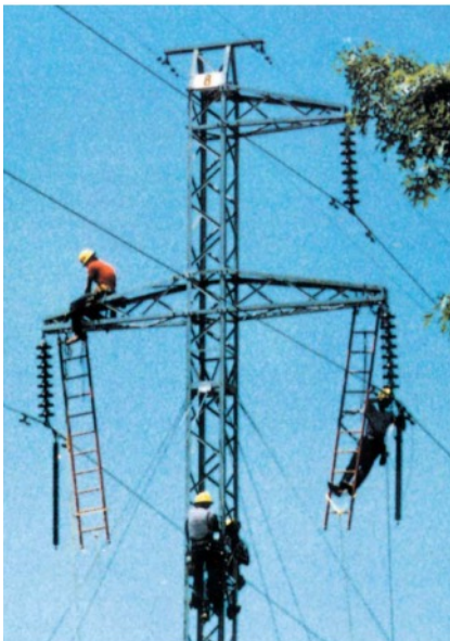
Figure 2: Installation of polymer housed NGLAs on 138kV circuit in late 1980s
